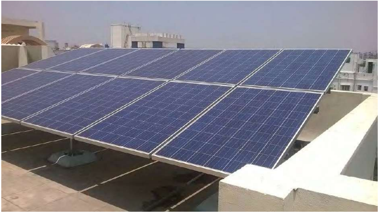
5KW on GRIDTIE SOLAR SYSTEM
